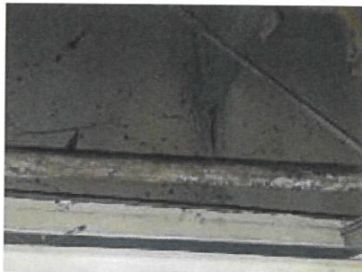
Dining Room/Living Room - Mold like substance on insulation above ceiling tiles
