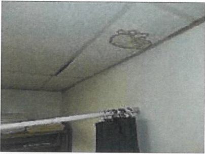
Men's Restroom - Water damaged ceiling Tile
