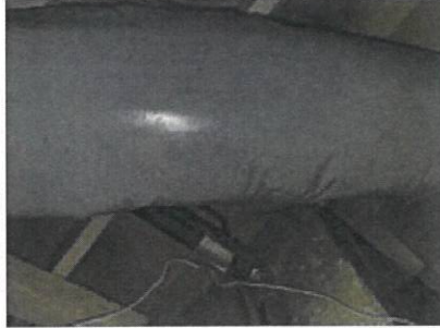
Washroom/Water Heater Closet - Mold like substance on ductwork
