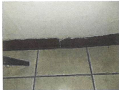
Women's Restroom - Mold like substance behind cove base
