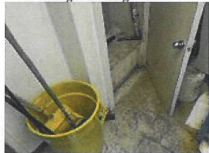
Washroom/Water Heater Closet - Mold like substance and water damage on HVAC stand
