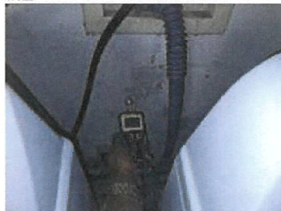
Washroom/Water Heater Closet - Elevated moisture on wall
