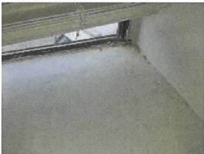
2nd Floor West Bedroom - Water damaged windowsill
