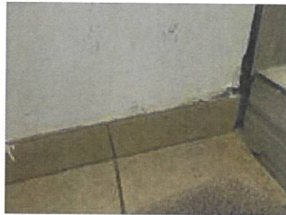
Men's Restroom - Water damaged lower wall
