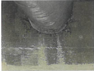
Washroom/Water Heater Closet - Mold like substance on HVAC unit
