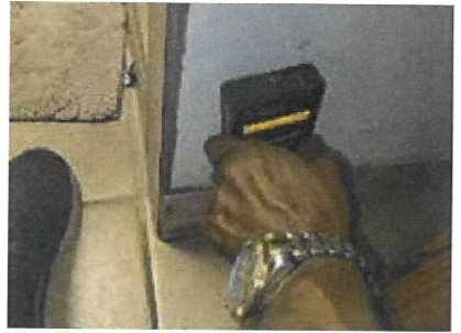
Men's Restroom - Elevated moisture on wall
