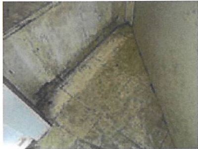
Washroom/Water Heater Closet - Mold like substance and water damage on HVAC stand
