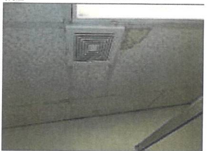
Men's Restroom m - Water damaged ceiling Tile
