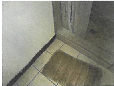
Women's Restroom - Water damaged lower wall
