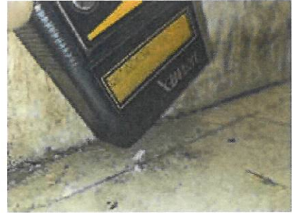
Washroom/Water Heater Closet - Elevated moisture on fwall
