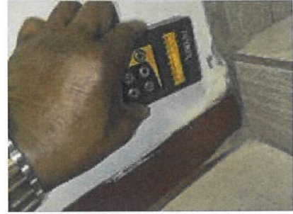
Women's Restroom - Elevated moisture on wall
