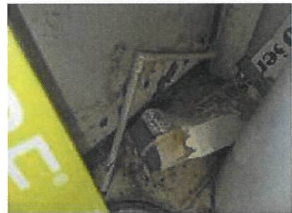
Washroom/Water Heater Closet - Mold like substance and water damage on wall
