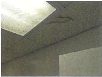
2nd Floor West Bedroom - Water damaged ceiling tile
