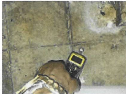
Washroom/Water Heater Closet - Elevated moisture on flooring
