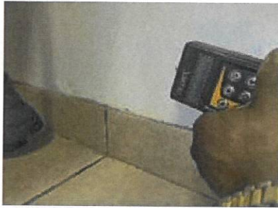
Men's Restroom - Elevated moisture on wall
