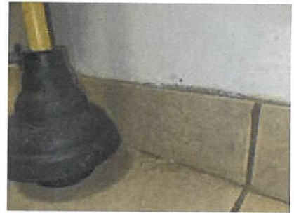
Men's Restroom - Water damaged lower wall
