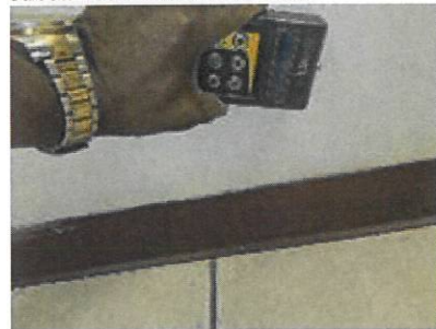
Women's Restroom - Elevated moisture on wall
