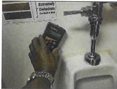
Men's Restroom - Elevated moisture on wall
