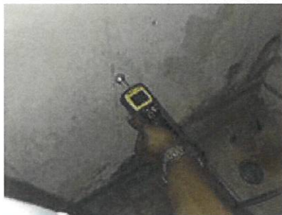
Washroom/Water Heater Closet - Elevated moisture on wall
