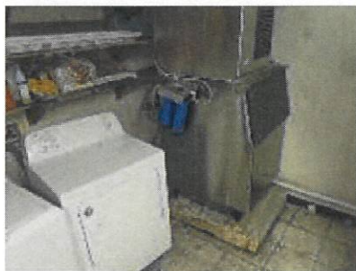
Washroom/Water Heater Closet
