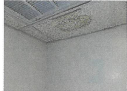
2nd Floor West Bedroom - Water damaged ceiling tile
