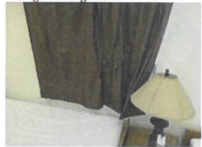
2nd Floor West Bedroom - Water damaged windowsill
