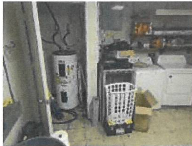
Washroom/Water Heater Closet
