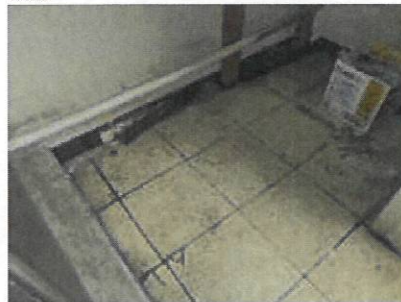
Washroom/Water Heater Closet - Water damaged flooring
