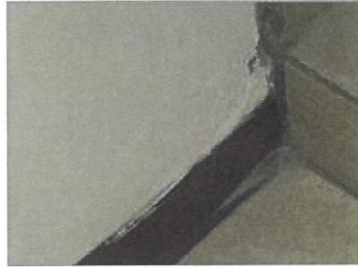
Women's Restroom - Water damaged lower wall
