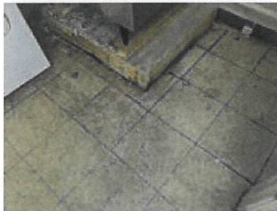
Washroom/Water Heater Closet - Water damaged flooring
