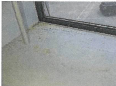
2nd Floor West Bedroom - Water damaged windowsill
