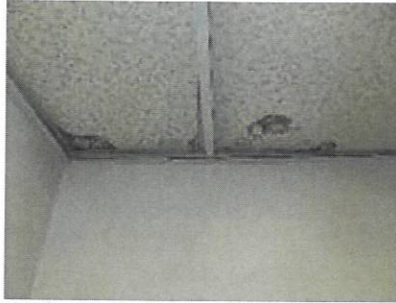
Dining Room/Living Room - Water damaged ceiling tile
