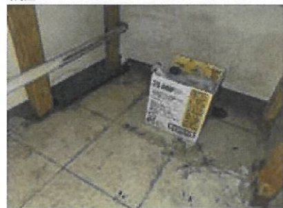
Washroom/Water Heater Closet - Water damaged flooring
